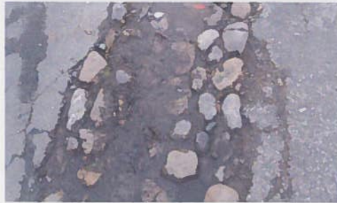
The distinctive cobble gully to the perimeter of the Market Place is being progressively eroded and would benefit from protection and enhancement. A level stone kerb to either side of the gully would provide a definitive 'stop edge' for the tarmac.
